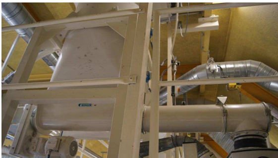
Hopper on top of MSDA
