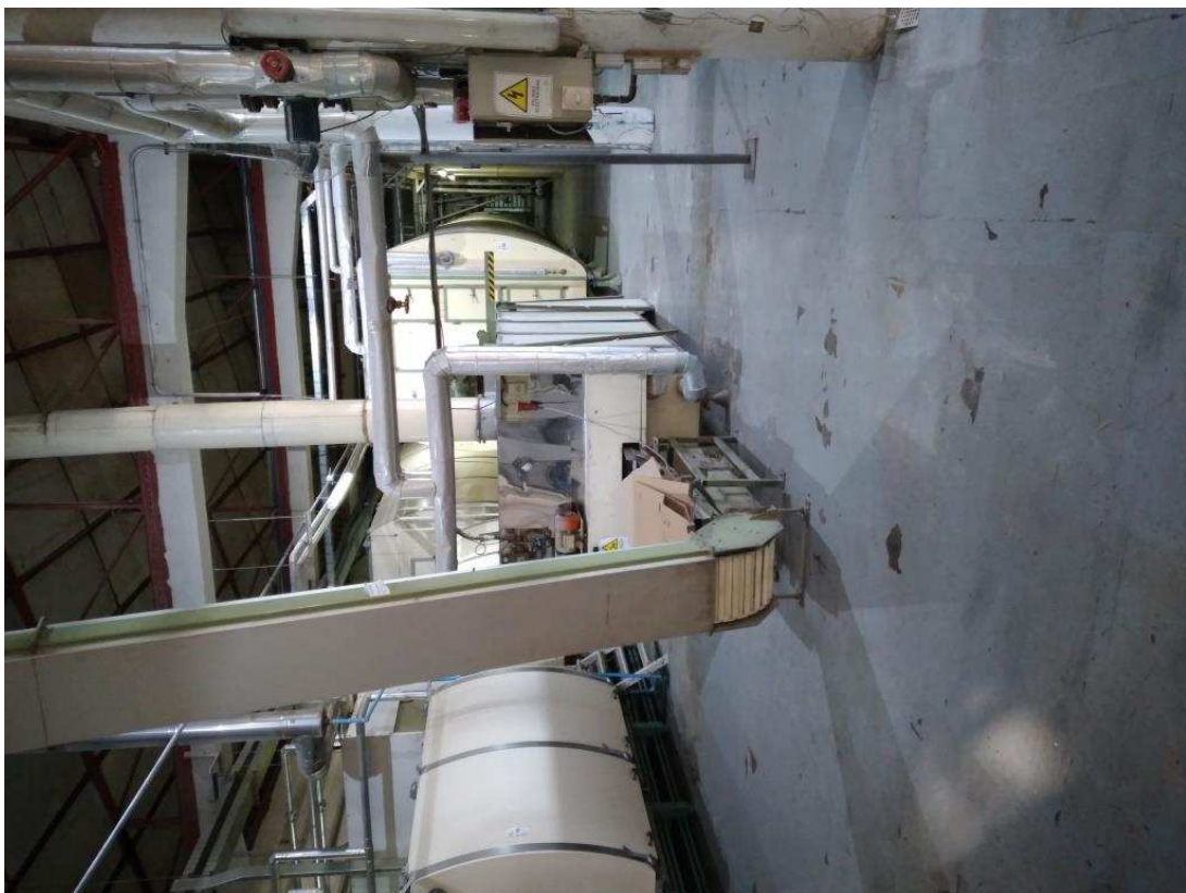
Cooler and Bucket Elevator
