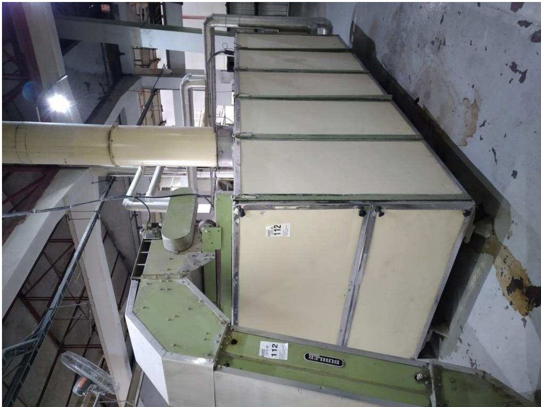
Bucket Elevator and Cooler
