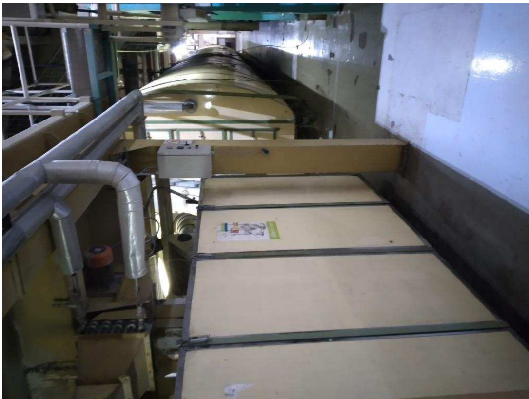
Shaker Pre Dryer
