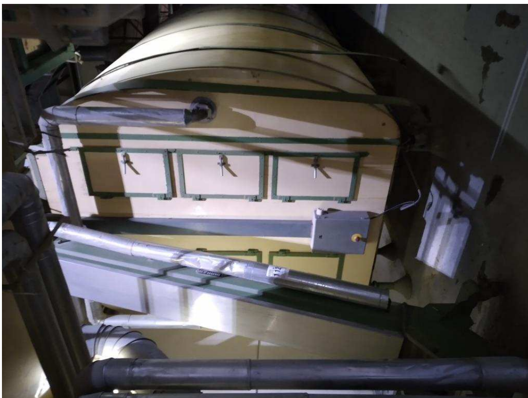
Heated Bucket Elevator in between Pre- and Final Dryer
