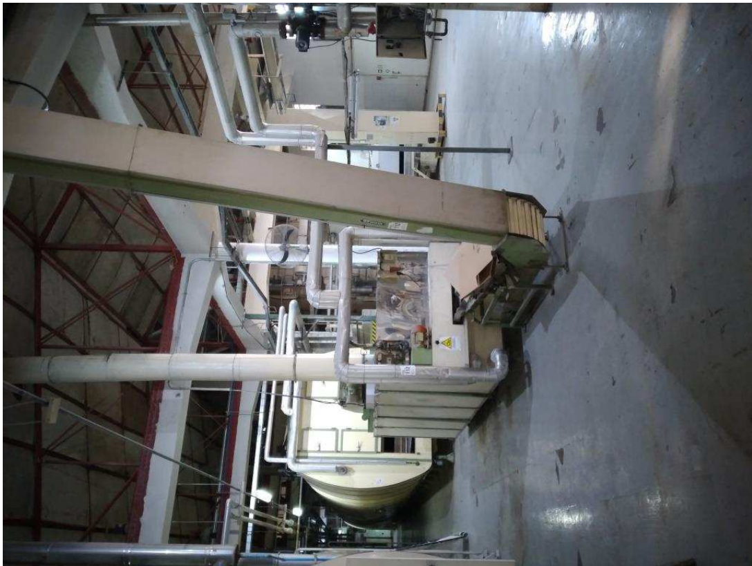
Final Dryer, Cooler, Bucket Elevator
