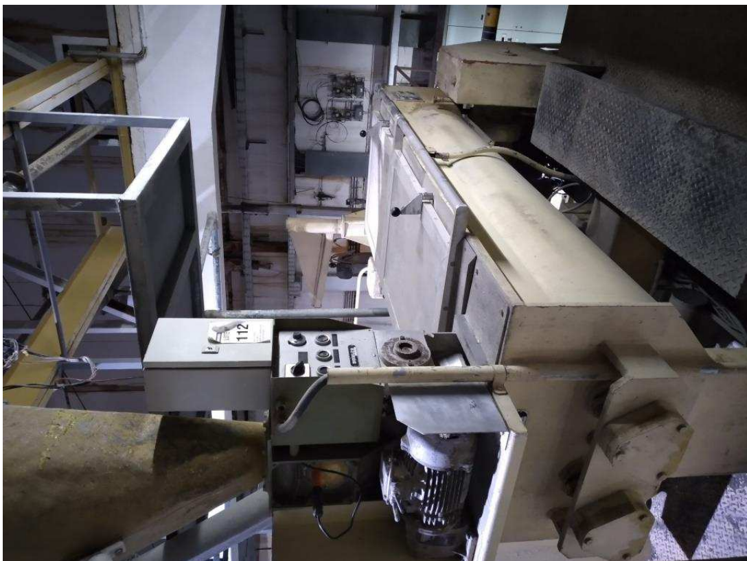
TCDS Dosing Unit and Main Mixer
