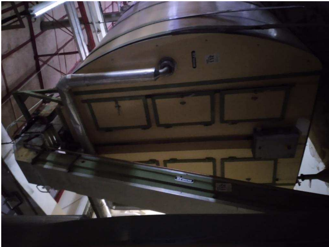
Intake Final Dryer
