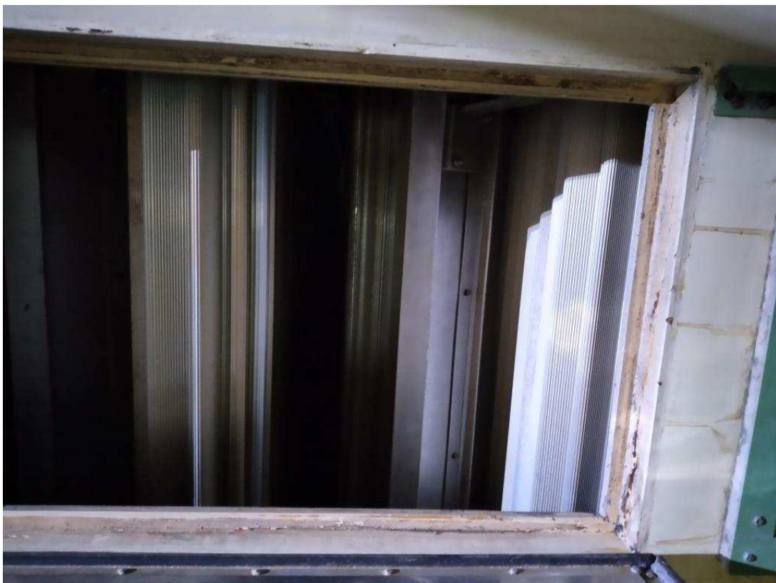
Opened Door at Final Dryer
